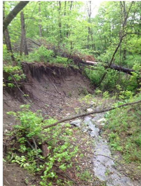
Figure C9. Stormwater that drains to the pictured gully from both the Health Center's detention pond outlet and from an unmanaged stormwater outfall. Significant erosion has occurred.
