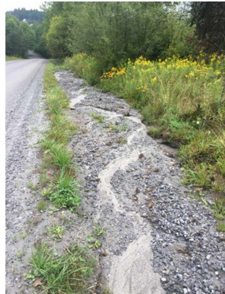
Figure C21. Sediment is clogging the roadside ditch on Middle Road.
