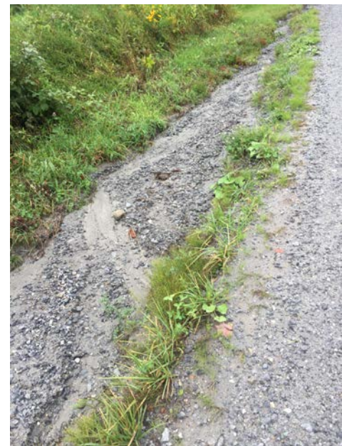
Figure C13. A section of Middle Road where roadside ditches are filled with sediment.
