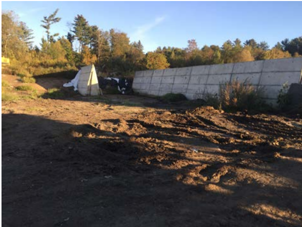
Figure B25. Unstable area at Neddo Farm.
